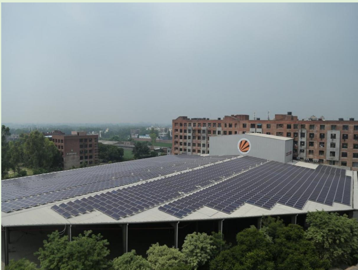
Solar Power Plant established on the rooftop
