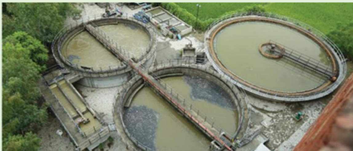
5 MLD Sewage treatment plant installed in Campus
