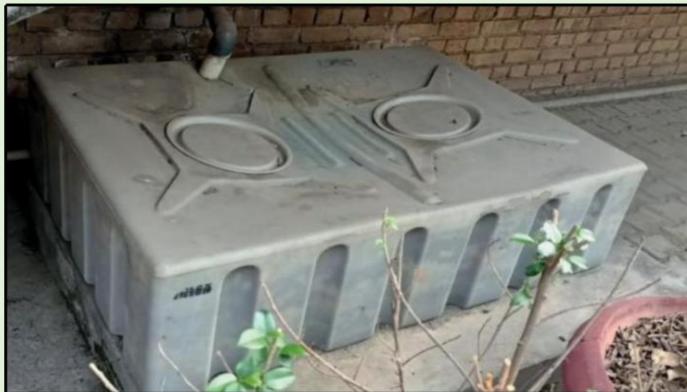
Loft water tanks installed to prevent the entry of polluted water into the broader water infrastructure
