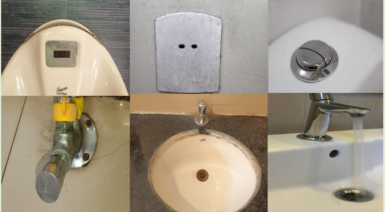
University replaced all traditional fixtures to reduce unnecessary water flow
