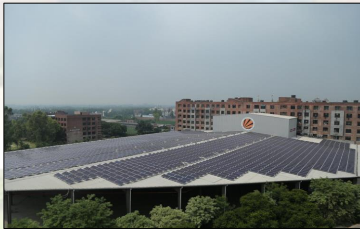
Solar Power Plant
