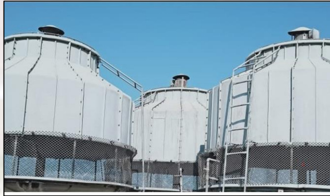
Centralized Chiller Plant
