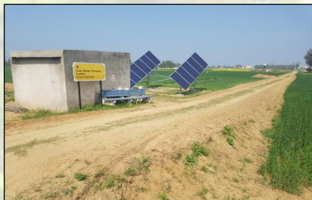
Solar Water Pumping system
