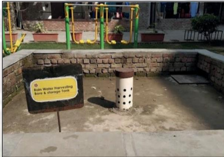
Rainwater Harvesting Bore at LPU
