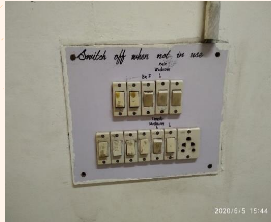
Well labeled switchboards
