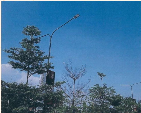
LED-based street lighting
